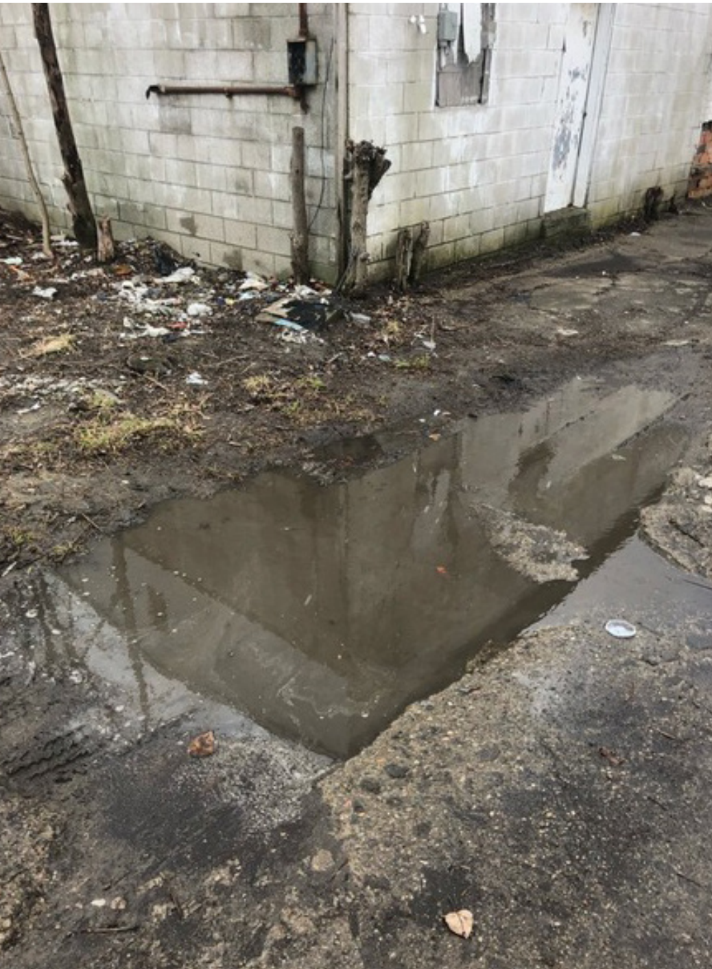
FIGURE 22. A BLOCKED CATCH BASIN IN DETROIT, AS REPORTED BY A HOMEOWNER. SOURCE: EN.SEECLICKFIX.COM.
