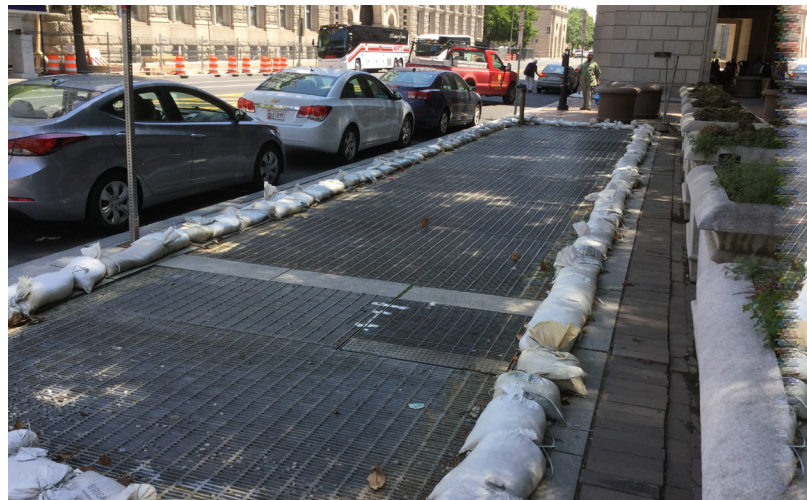
FIGURE 31. SANDBAGS BLOCKING STORMWATER FLOW FROM WASHINGTON METRO SUBWAY AIR VENT. SOURCE: G. GALLOWAY, UMD.
